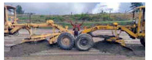
Cory Bell seen with the twin road graders that help keep the Northport International Raceway track surface race ready. Northport photo
